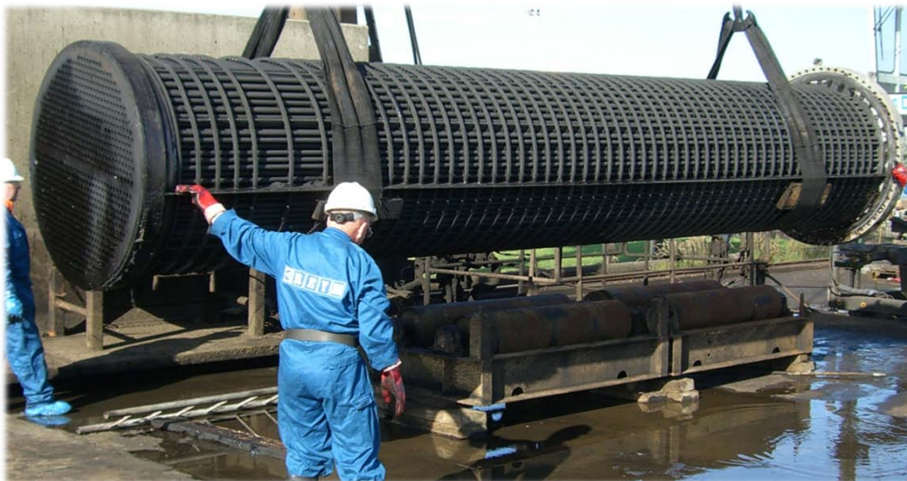
EMbaffle® bundle before cleaning, showing no particulate fouling or 'dead zones'
